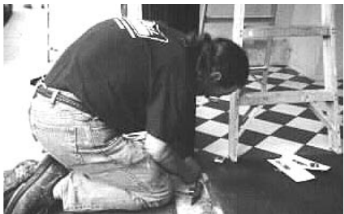
The function of a set of modern metal framed doors (below) is being restored by replacing the pivots which have failed due to corrosion.
