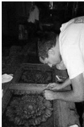
A Dell Preservation Technician (right) works to restore the form of an original set of 19th century oak doors by removing years of paint and varnish.
